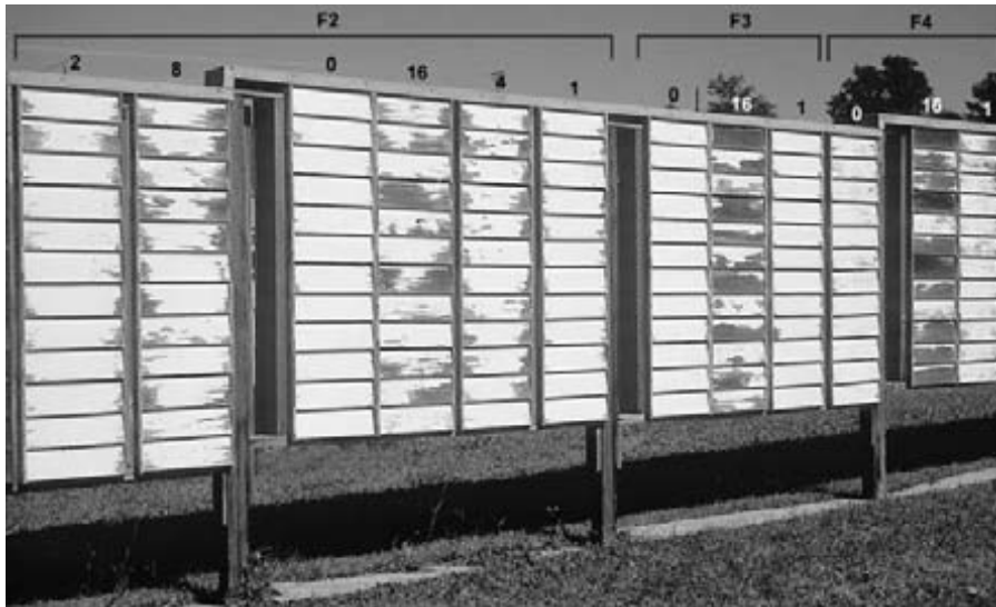
Figure 1 (Facing page): Paint failure on an eight-year-old structure left unpainted for several months following construction. Failure following the third time the structure was painted is shown.
